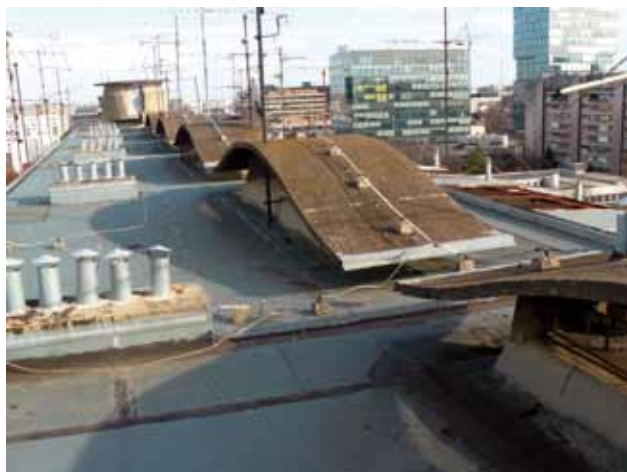
30 Vukovarska 35-35 a, krovna ploha (fototeka GSKG) Vukovarska 35-35 a, roof surface (photo archives of GSKG)
