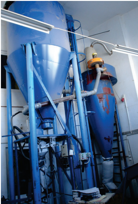
Figure 1 Mixing line in an industrial feed plant in the following unit: a feed mixer, an intake hopper and a bucket conveyor
