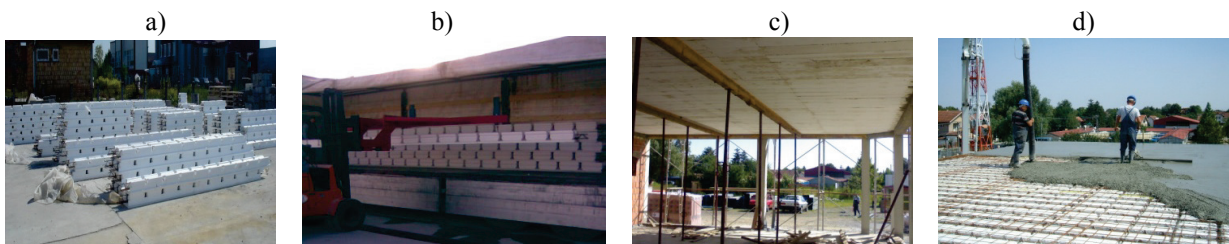
Figure 10 a) Production of StiroFert beams, b) loading the truck bed StiroFert, c) Installation of StiroFert beams on construction site, d) Concrete slab on the site
