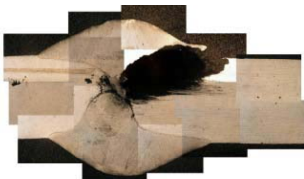
Figure 6. Presentation of a real corrosion damage initiated at the fusion line of AISI 304L welded joint caused by microbiologically influenced corrosion in form of pitting (water tank, 3 months in use, thickness of the base material: 4 mm)
