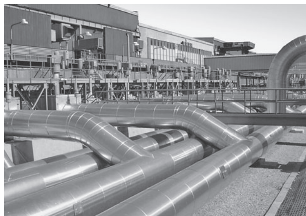
Figure 1 Part of a technological system of a compressor station for gas transport
