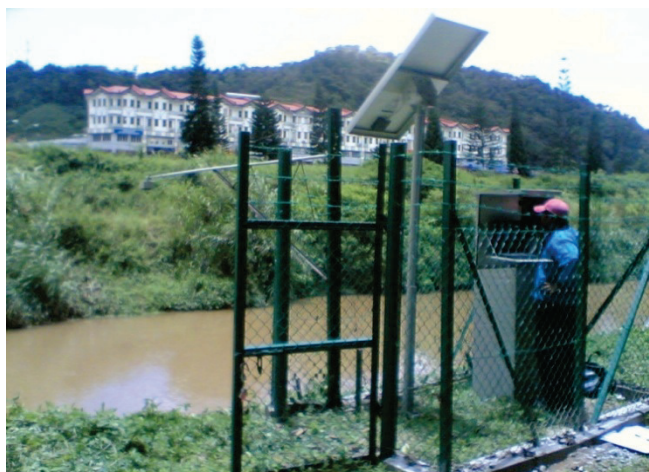
Figure 3 River discharge and water level automatic recording station
