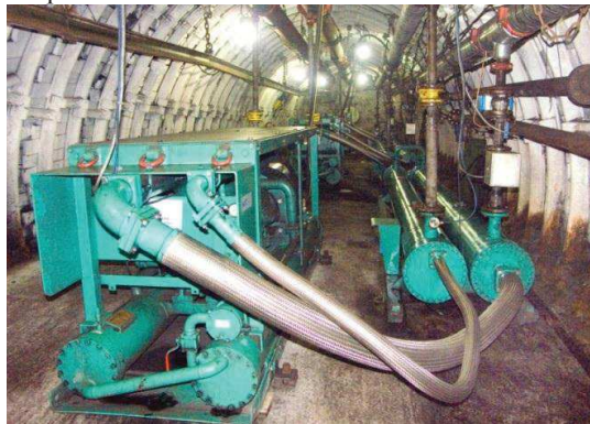
Figure 5 Arrangement of the cooling equipment in mine machine room
