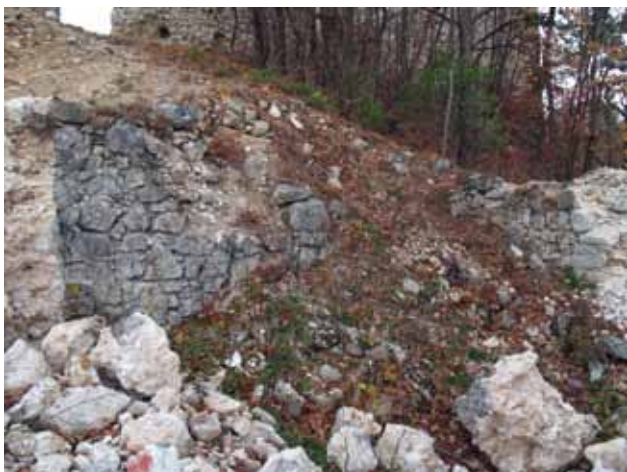
21 Pogled na sjeverni zid i urušeni dio zapadnog zida kapele utvrde Grebengrad, stanje 2009. (foto: M. Korunek) View of the northern wall and collapsed part of the western wall of the chapel of Fort Grebengrad, condition in 2009 (photo: M. Korunek)
