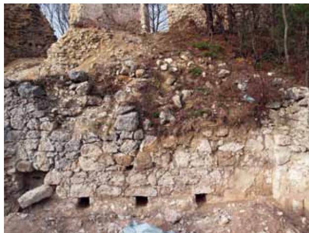
22 Sjeverni zid kapele utvrde Grebengrad, unutrašnjost, stanje tijekom radova 2012. (foto: M. Korunek) Northern wall of the chapel of Fort Grebengrad, interior, condition in the course of works in 2012 (photo: M. Korunek)
