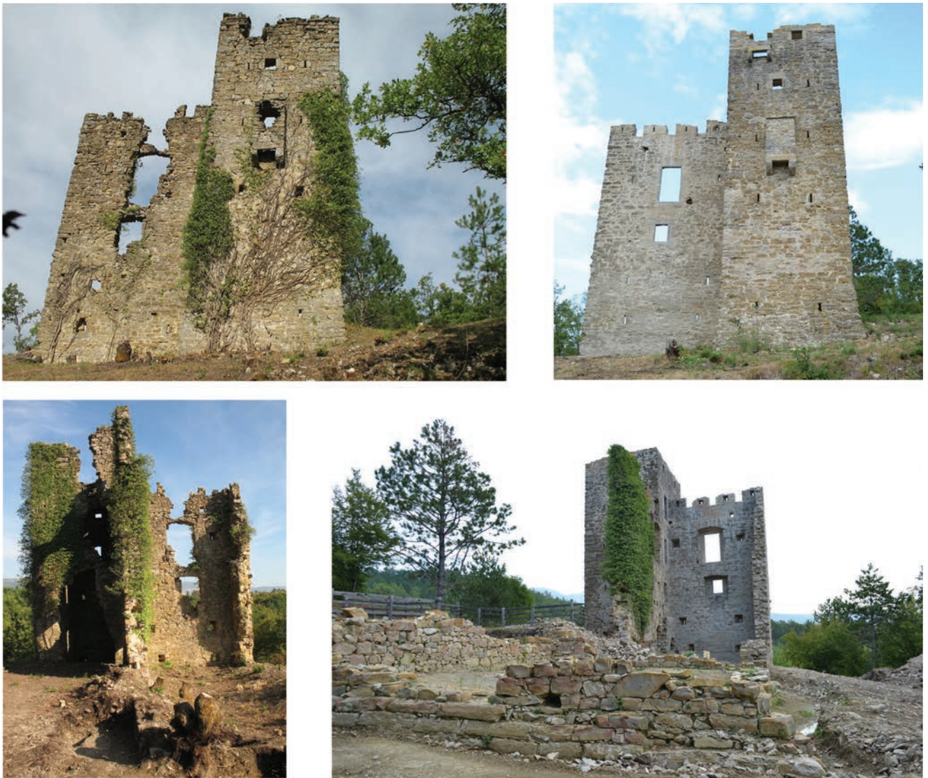
Sl. 10 Primjeri stanja zidova utvrde prije i poslije konzervatorsko-restauratorskih radova. Fig. 10 Examples for the state of the walls of the fort before and after the conservation-restoration works.
