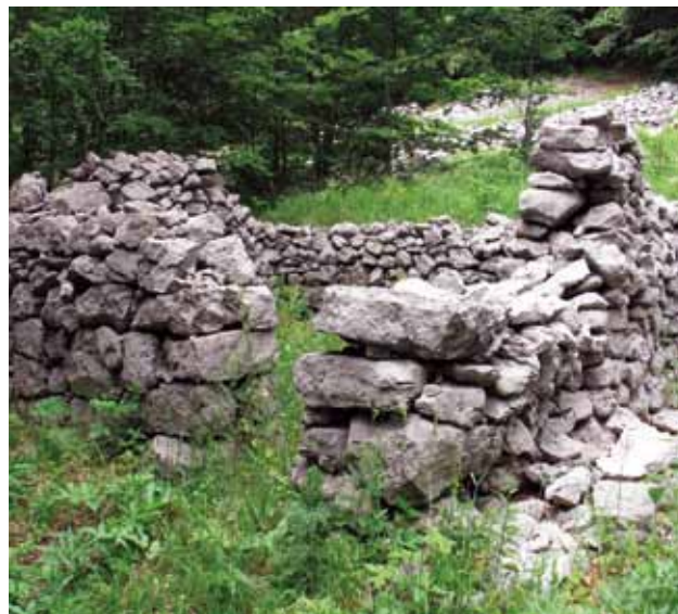
10 Ruševina pastirskog stana na Alanu (foto: M. Ivanuš) Ruin of shepherd's dwelling on Alan (photo: M. Ivanuš)
