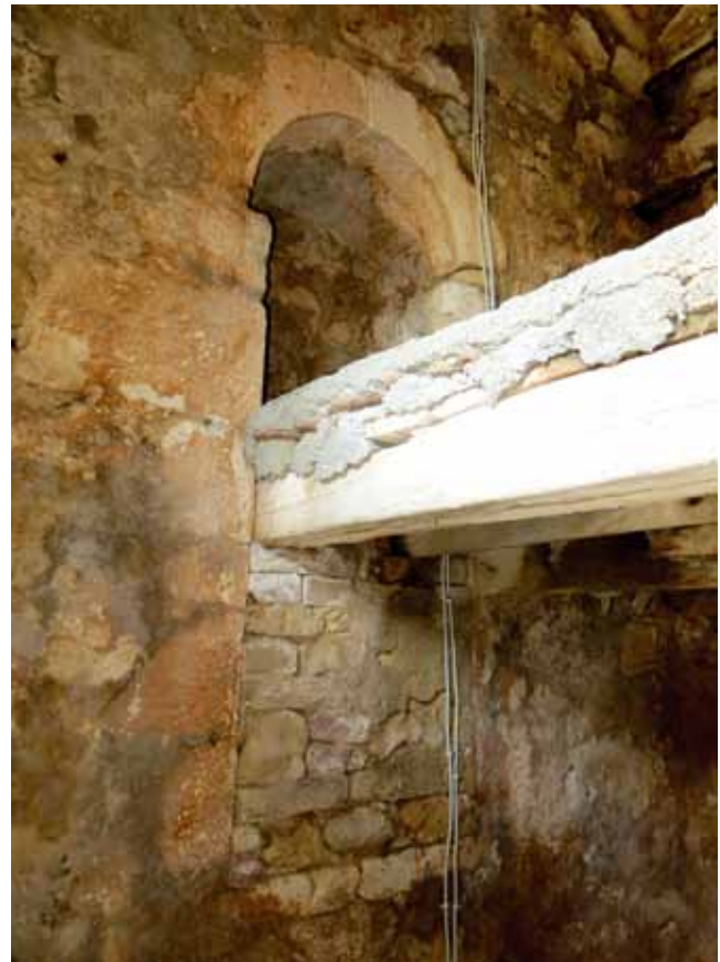
4. Zazidana monofora istočne stranice trećeg kata zvonika (foto: E. Motušić) Walled-up single-light window on the east side of the third floor of the bell tower
