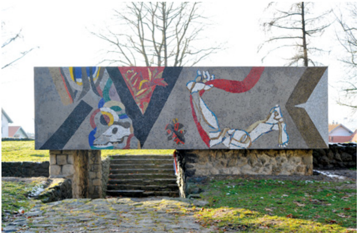
16. Pogled na mozaik koji se nalazi na istočnom zidu, nakon radova 2012. (snimio J. Kliska, Arhiv HRZ-a). View of the mosaic on the eastern wall, after the conservation in 2012 (photo by J. Kliska, Croatian Conservation Institute Photo Archive)
