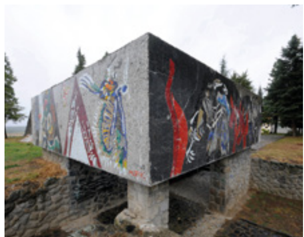
10. Pogled na jugozapadni ugao spomenika, prije radova 2012. (snimio J. Kliska, Arhiv HRZ-a). View of the southwestern corner of the monument, prior to conservation in 2012 (photo by J. Kliska, Croatian Conservation Institute Photo Archive)
