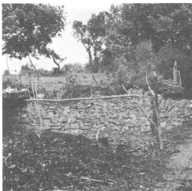
T. 11, 3 Detalj istočnog zida kvadratne kule kastrona. Danas je ovdje tor za stoku. Snimio: Ž. Tomičić (1988). Detail of the eastern wall of the rectangular tower of the fort. Today it is a cattle pen.
