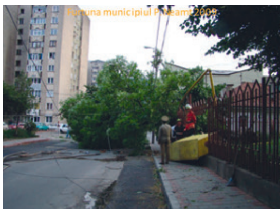
Figure 2. Material losses produced by strong winds during a storm, Piatra Neamț, 2009
