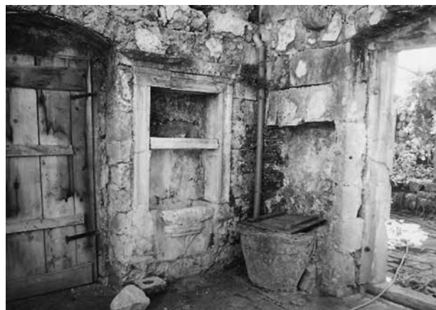
2. Ladanjsko-gospodarski kompleks Crijević-Lobro, Radovčići, zidni umivaonik u prizemlju / The residential-farming complex Crijević-Lobro, Radovčići, wall wash-basin on the ground floor
