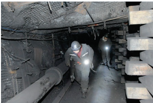
Figure 9 Severe roof-to-floor convergence in the cut-through entry at which conventional wood cribs were installed
