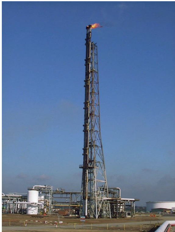
Figure 1: Flare stack at refinery
