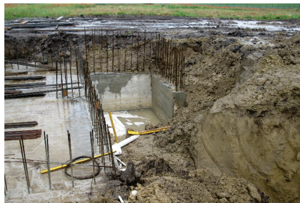
Figure 2 Saturation and sliding ground around the foundation pit
