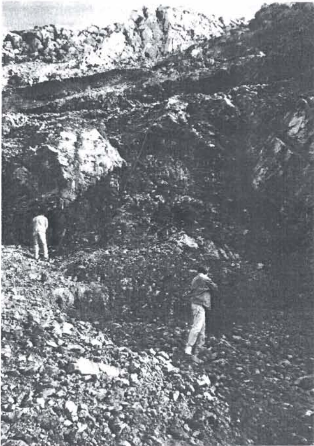
Fig. 6. Excavation for the arch foundations on the east side of Novsko ždrilo
