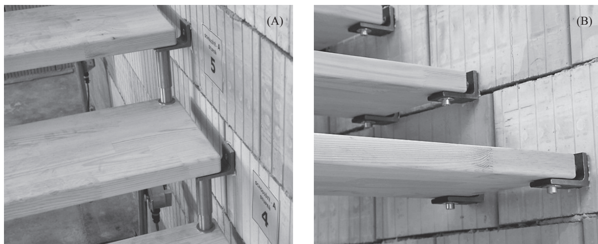
Figure 6 Different ways of fixing the stairs into the bearing wall: (A) Version A (the stairs supported by a steel profile and by a distance element); (B) Version B (the stairs supported by two steel profiles)
