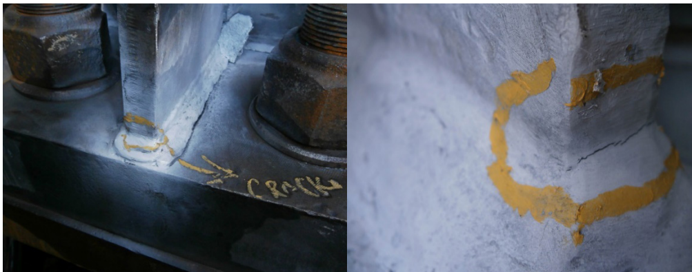
Figure 2. Cracks on derrick footing after 20 years usage.
