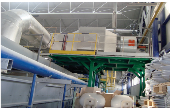
Figure 3 Heat exchanger inserted into channel and Heat exchanger installed on tunnel kiln
