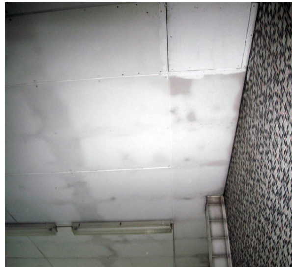
Figure 2 Asbestos boards on the ceiling of the Zasavje swimming pool facility where the patient worked in the 1970s
