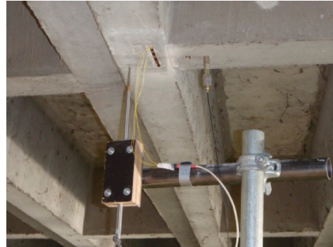
Fig. 11. Sensors under the Pernica Bridge.
