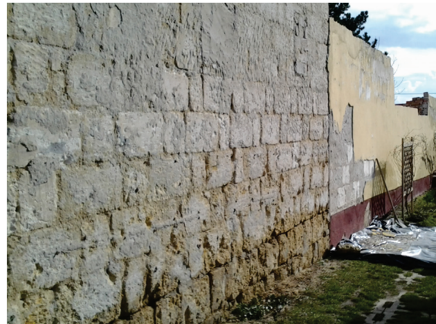
Figure 1 Moisture damaged coarse soft limestone masonry wall
