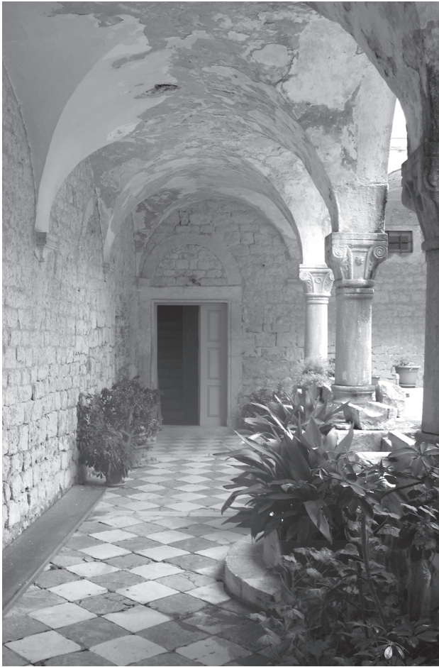
Samostan sv. Križa na Čiovu - istočno krilo klaustra / Monastery of the Holy Cross - eastern wing of the cloister
