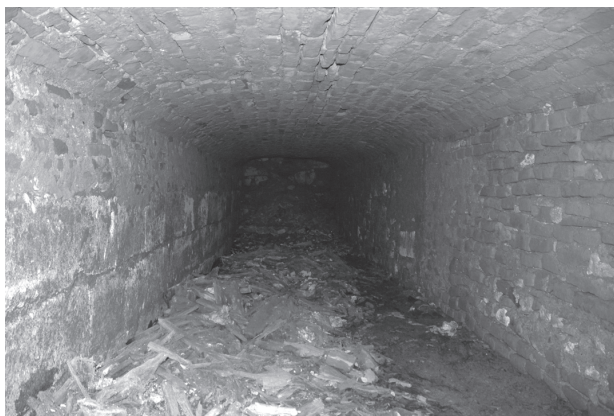
13. Kripta ispod zapadnog dijela cinktora (foto: Petar Puhmajer) / The crypt underneath the western section of the porch (photo: Petar Puhmajer)
