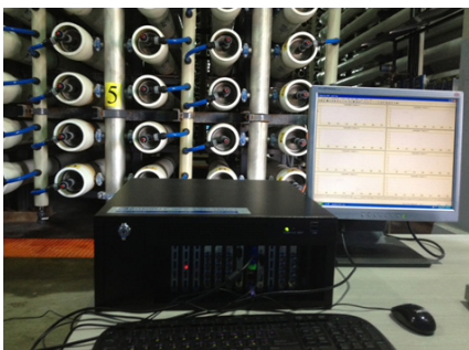
Figure 3. AE monitoring of several FRP vessels.
