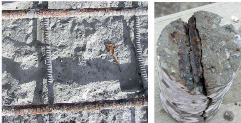
Figure 1. Exposed corroded rebars (left) and a corroded rebar extracted with a core (right).
