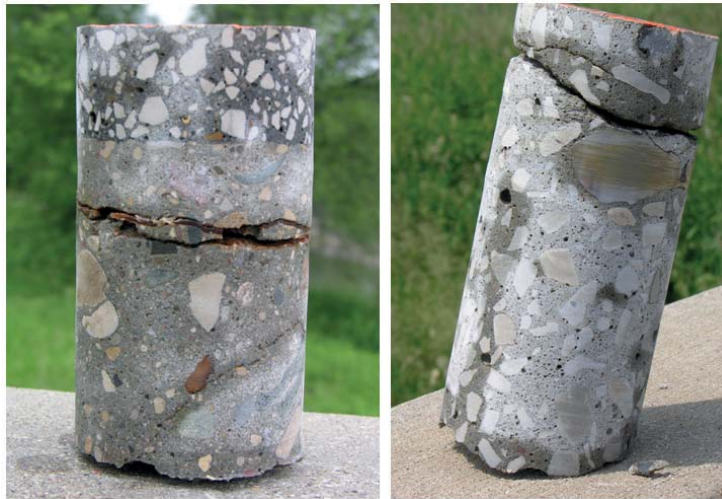
Figure 3. Cores extracted from delaminated bridge decks.
