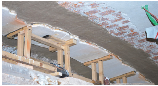
15. Detalj fragmenta nakon žbukanja armature mrežice (snimio M. Jelenčić, 2010.) Detail of the fragment after plastering the armature grid (photo by M. Jelenčić, 2010)
