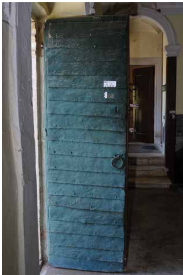
13. Vratnice predvorja u prizemlju (Dokumentacija HRZ-a, snimila: E. Šurina, 2013.) / Door panels of the ground floor hall (Documentation of the Croatian Conservation Institute, photo: E. Šurina, 2013)
