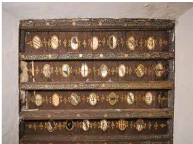
18. Dio oslikanog grednika jugozapadne prostorije kata (Dokumentacija HRZ-a, snimila: N. Vasić, 2013.) / Section of painted wooden ceiling of the southwest room of the first floor (Documentation of the Croatian Conservation Institute, photo: N. Vasić, 2013)
