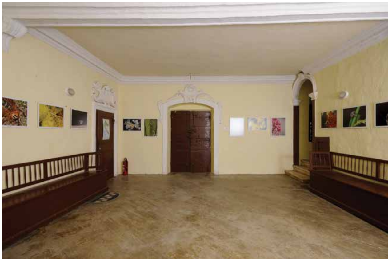
12. Predvorje prizemlja ukrašeno štukaturom (Dokumentacija HRZ-a, snimila: N. Vasić, 2012.) / Ground floor hall with stucco decorations (Documentation of the Croatian Conservation Institute, photo: N. Vasić, 2012)
