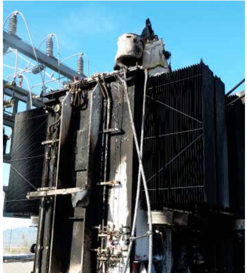
Figure 10. Catastrophically failed 500 kV transformer
