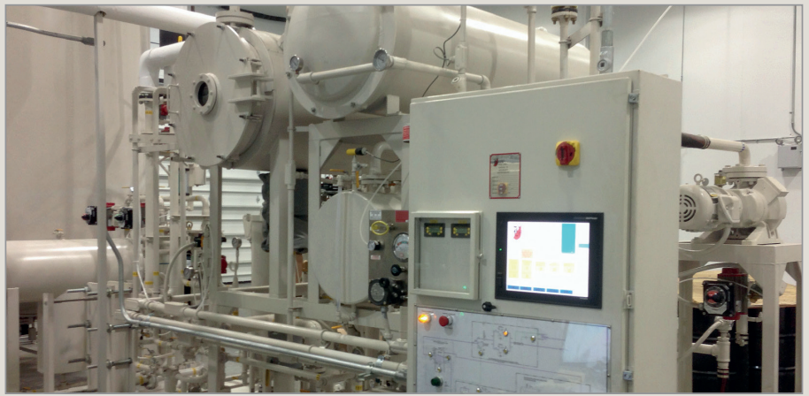
Figure 12. Vacuum Distillation Unit for solvent (VDU)
