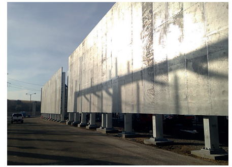
Major US substation protected by UL 752 Level 8 ballistic fire barriers installed to NFPA 851 Line of Sight
