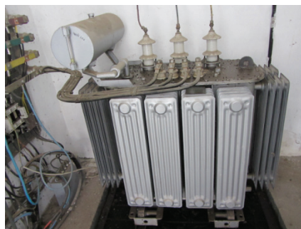
Figure 1 10/0,4 kV power transformer
