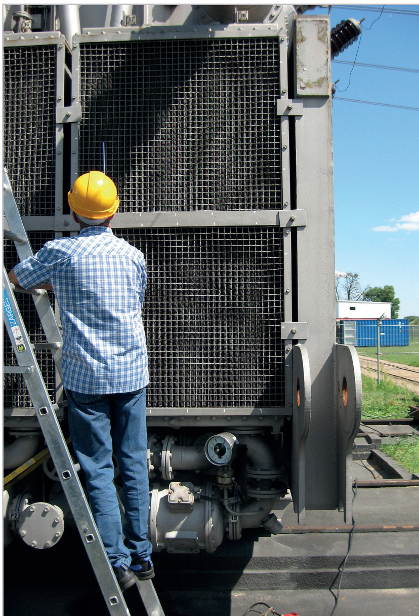
Figure 4. Measurement of noise emitted by the transformer oil cooler at a distance of 2 m. Replacement of these old fans by new fans with EC drive and advanced fan blade geometry lowered the sound level by 16 dB (A) and reduced power consumption.
