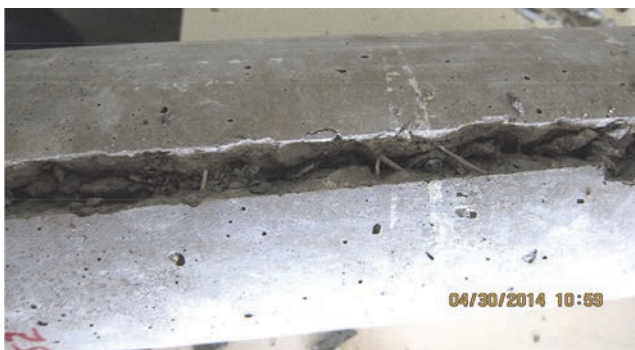
Figure 6. Fibres in concrete across crack section
