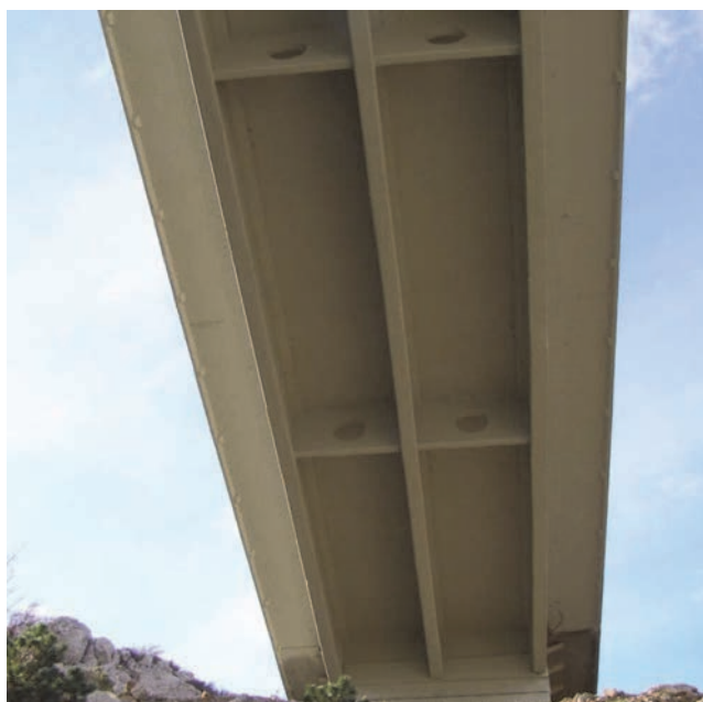
Figure 15. Deck slab bottom contour in the U5-S31 zone after application of the final coat of paint [14]
