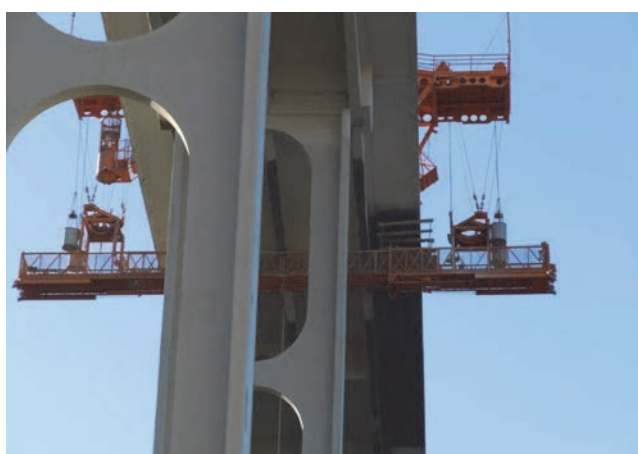
Figure 16. Deck slab bottom contour – S31-S30 zone - application of the final coat of paint [14]
