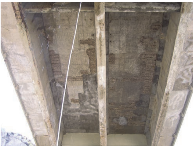
Figure 13. Bottom contour at the first third of deck slab in the U5-S31 zone after removal of damaged concrete [14]
