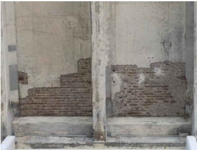
Figure 11. Deck slab bottom contour in the S31-S30 zone next to pier S31, moisture due to seepage at joint after hydrodemolition of damaged concrete [14]
