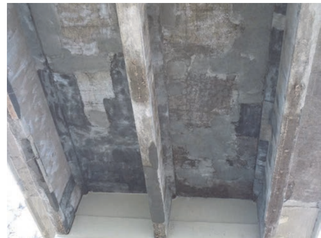
Figure 14. Bottom contour at the first third of deck slab in the U5-S31 zone after placement of the repair system [14]
