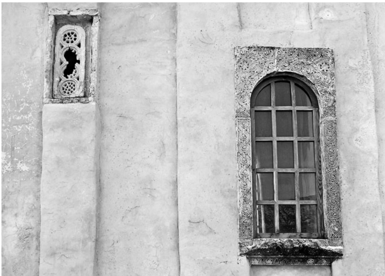
5. Crkva Sv. Mihajla, Ston, tranzena i prozorski okvir, sjeverna strana (foto: P. Marković, 2011.) St Michael's church in Ston, transenna and the window frame, northern side
