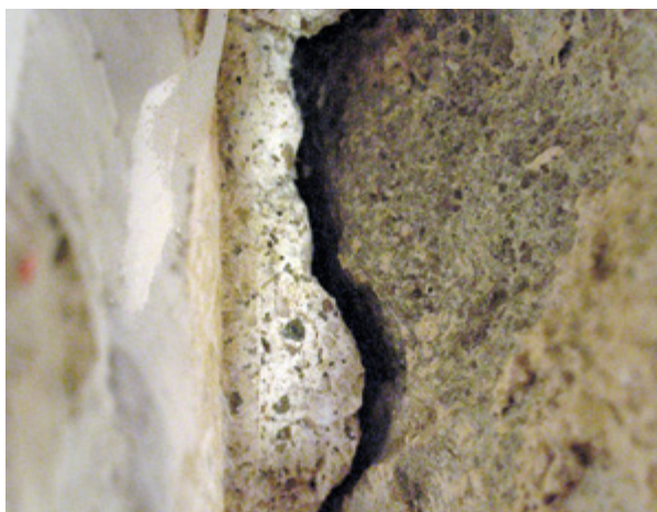
5. Šupljina, odvajanje arriccio od nosača (snimio B. Hacker, 2009.) A cavity, arriccio detaching from the support (photo by B. Hacker, 2009)
