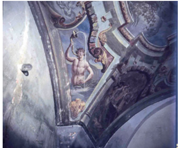
9. Detalj freske na jugozapadnoj peti svoda s vidljivim oštećenjima slikanoga sloja 1979. godine (Arhiv RZH-a, snimio I. Maroević) Detail of the fresco on the southwest foot of the vault with visible injuries to the painted layer in 1979 (former Conservation Institute of Croatia archive, photo by I. Maroević)
