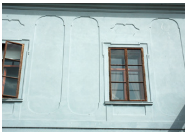
23. Osijek, Gradski magistrat, detalj pročelja (snimio P. Puhmajer, 2015.) Osijek, Old Town Hall, façade detail (photo by P. Puhmajer, 2015)
