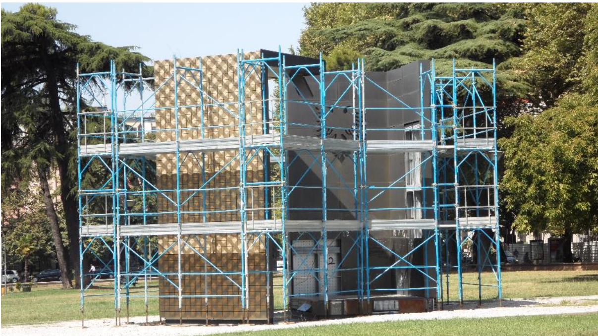
Figure 4. The scaffolding surrounding the Tirana Independence Monument, photographed in summer 2015. Photo by the author.
