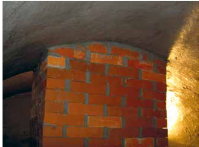
9 Novoizvedeni stup u cisterni (foto: I. Šprljan) Newly executed pillar in the cistern (photo: I. Šprljan)
