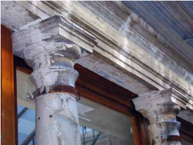
7 Pročelje, drugi kat, stanje stupova prije radova (foto: I. Šprljan) Frontispiece, 2 nd floor, condition of pillars prior to works (photo: I. Šprljan)
