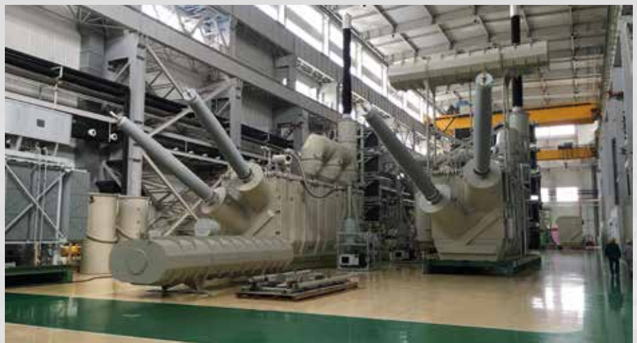
Transformers Magazine team (Mladen Banovic, Jason Song and George Jiang) visited SPECO, world's largest transformer factory, in Jinan, China, for the second time in one year, October 2016
