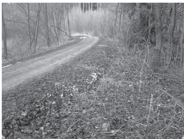
Fig. 6 The implemented reinforcement using brown chips with a cover layer of vibrated gravel
