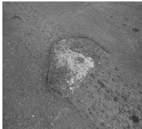
Fig. 8: Medium-severity potholes in Sample No. 278, Al-Fiush Road.
