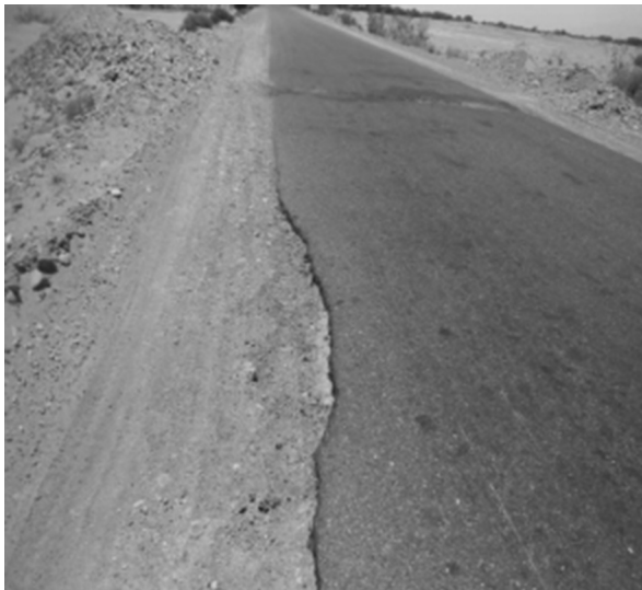
Fig. 7: High-severity edge cracking in Sample No. 278, Al-Fiush Road.
