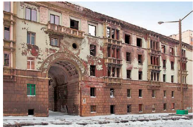
Figure 6: Unfit building at Bogdan-Khmelnitzkiy Street
