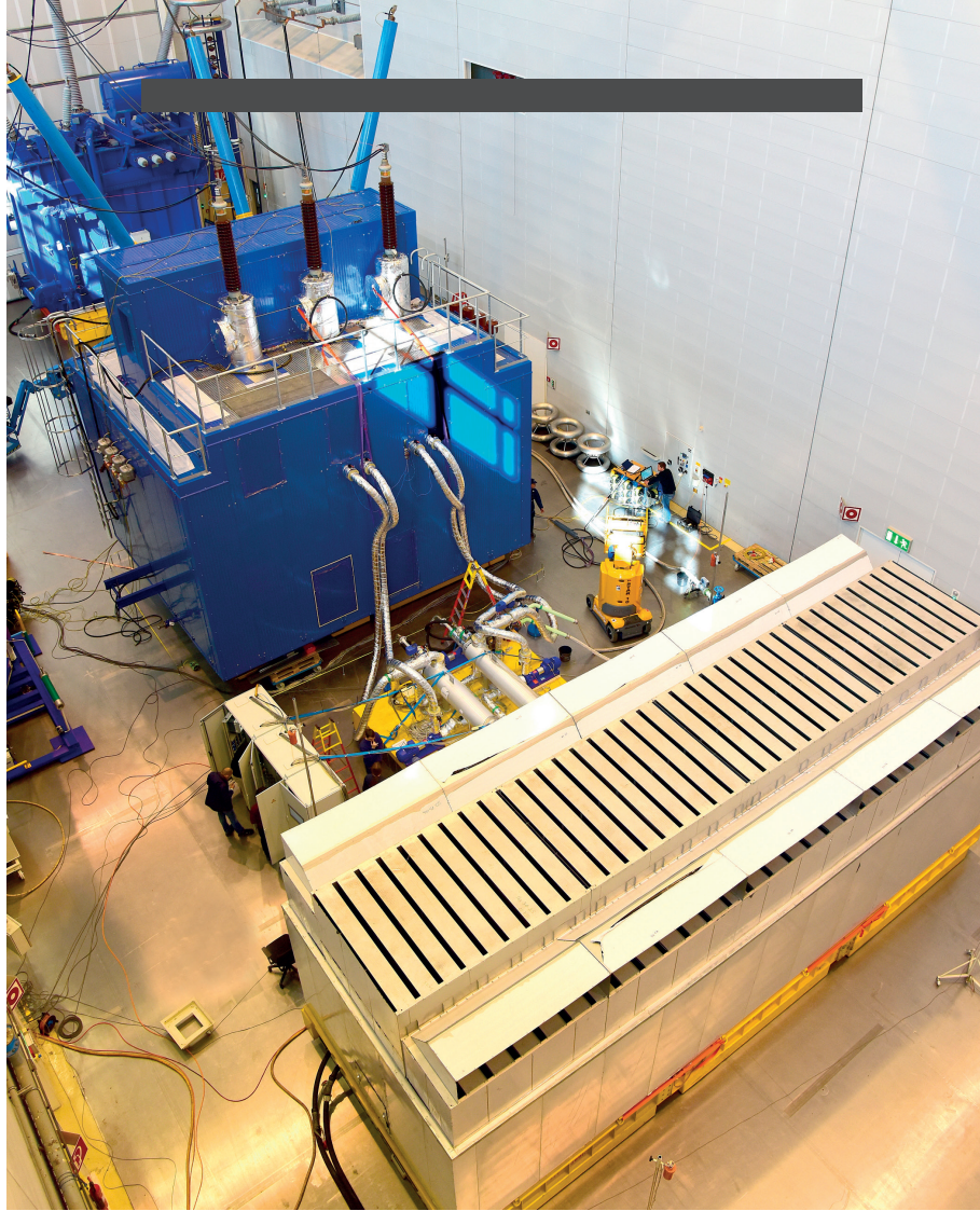
Figure 6. Transformer cooling system (heat exchanger) special silencers in the test bay
