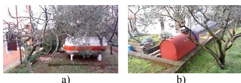
Figure 12 Fuel storage tanks: photos by A. Poropat, a) gas tank, Kovači (09.02.2016.); b) oil tank, Poreč-Hospital (12.02.2016)
