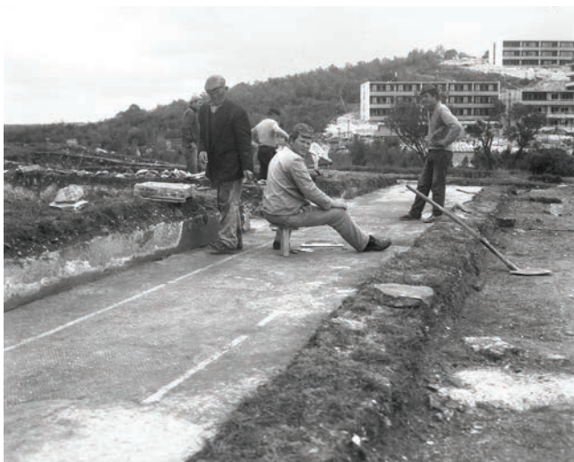
Sl. 18 Mozaik u hodniku istok-zapad tijekom zahvata konzervacije. Vidljiv je i detalj zida s obojanom žbukom (foto arhiva Arheološkog muzeja Istre). Fig. 18 The mosaic in the east to west corridor in the course of the conservation intervention. Also visible is a detail of the wall with painted plaster (photographic Archives of the Archaeological Museum of Istria).
